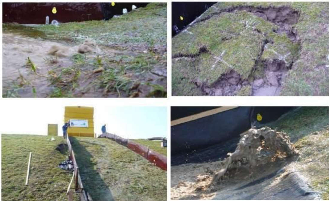
Figure 6-12: Rapid failure because of internal erosion and undermining of the grass cover at a wave overtopping test site with a combination of fragmented grass sod and a thin clay layer
